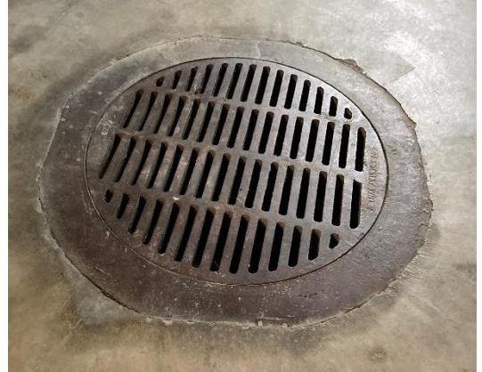
Figure 17: Garage Catch Basin
