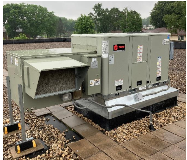
Figure 6: RTU-2, Trane Rooftop Air Handling Unit.
