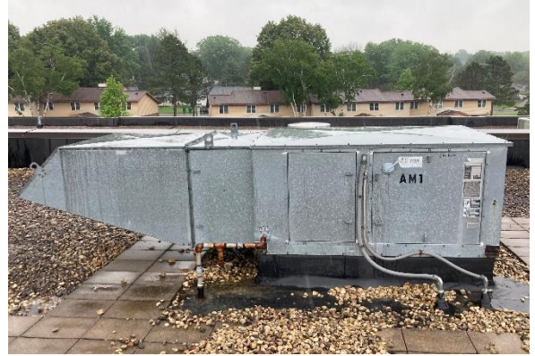
Figure 5: MAU-1, Fire Garage Make Up Air Unit.
