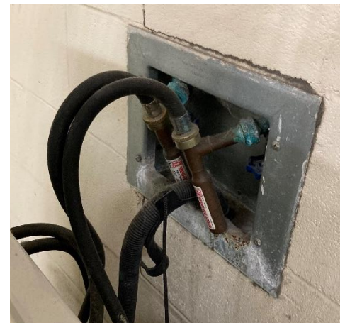
Figure 15: Visible Corrosion Example, Washer Box
