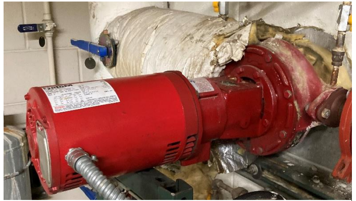
Figure 8: Pump P-1, Bell and Gossett Hydronic System Circulation Pump
