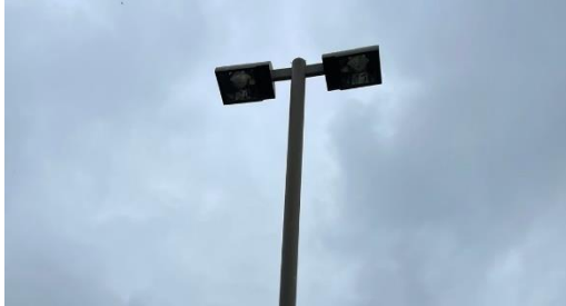
Figure 21: Existing Outdoor Light Pole
