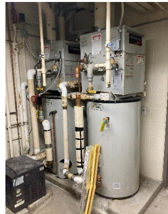
Figure 13: GWH-1,2 Decommissioned Water Heaters
