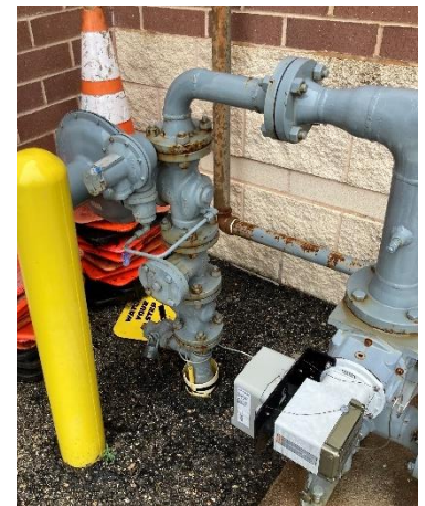
Figure 16: Rusting Gas Meter
