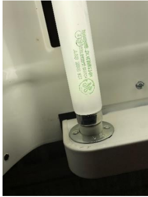
Figure 18: Existing Fluorescent Tube
