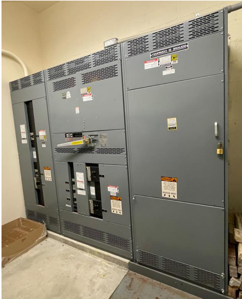
Figure 23: Existing Service Entrance Equipment
