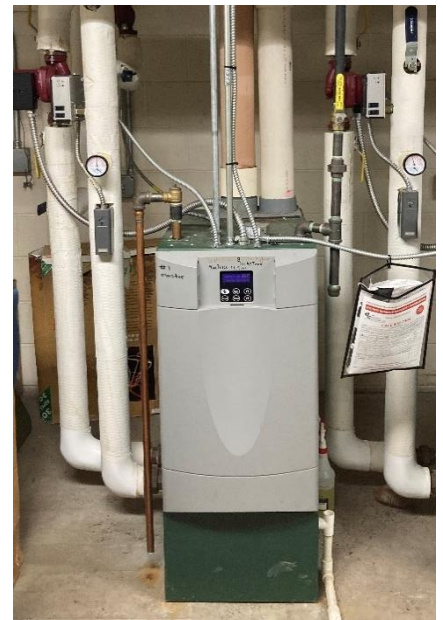
Figure 10: Peerless Boiler B-1
