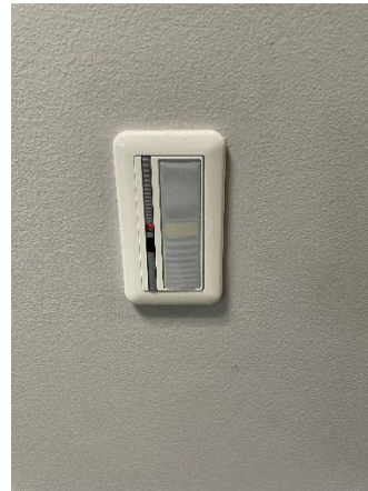
Figure 20: Existing Wall Occupancy Sensor
