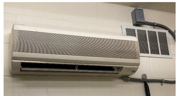
Figure 12: Mitsubishi Split System Heat Pump
