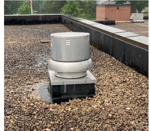
Figure 4: EF-5, visible corrosion. Carnes Downblast Exhaust Fan.
