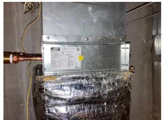
Figure 2: Hot Water Coil for VAV-4.02
