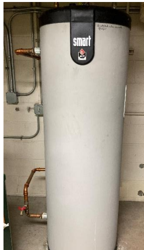
Figure 14: GWH-3, Operational Water Heater
