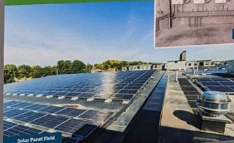
Solar Panel Field
