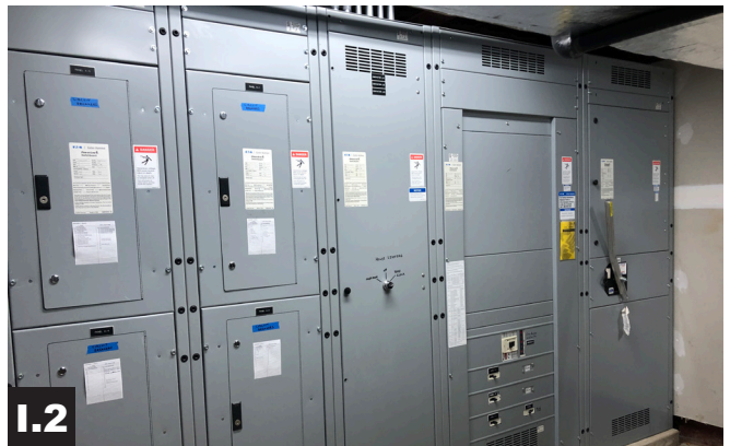
I.2 Electrical: Electrical is currently within the same area as mechanical and will be challenging to expand.
