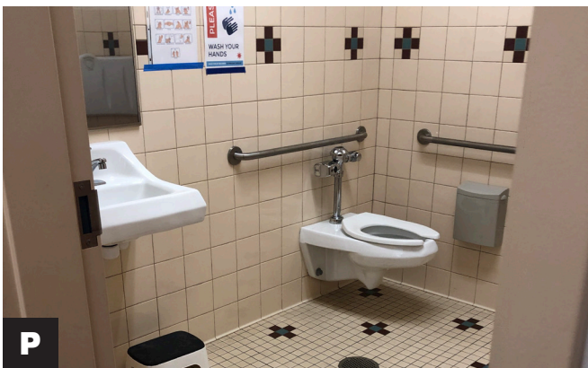
P Restrooms: The restrooms appear to be outdated, although fixtures appear to be in good working order. Newer sustainable measures could be provided along with individual restrooms for staff and children & families.
