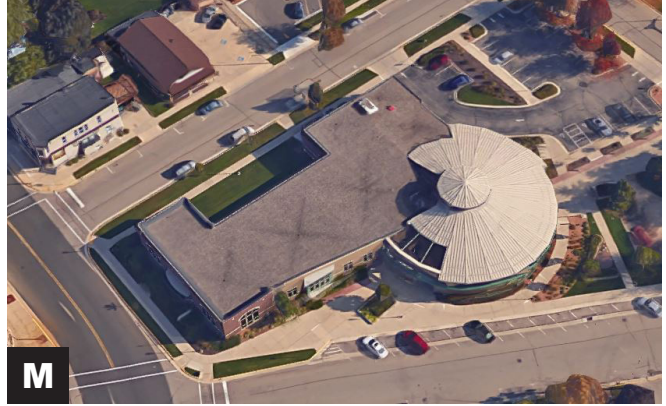
M Roof: The overall condition was not fully reviewed at the time of this report. Indications from staff were that the roof was in good shape.
