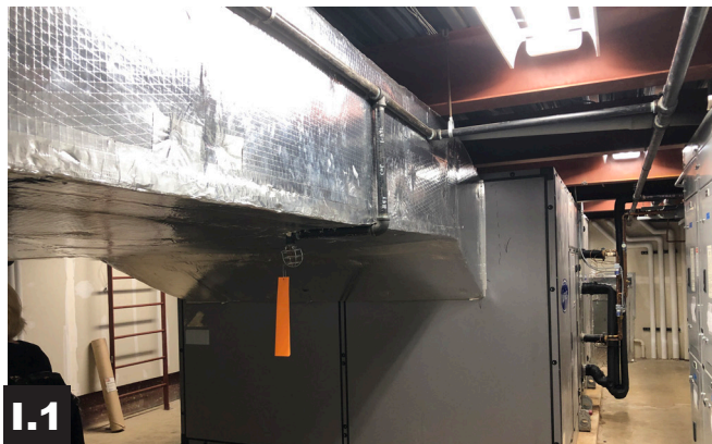
I.1 Mechanical: Mechanical is currently on a mezzanine within the staff area. Access and expansion will be limited.
