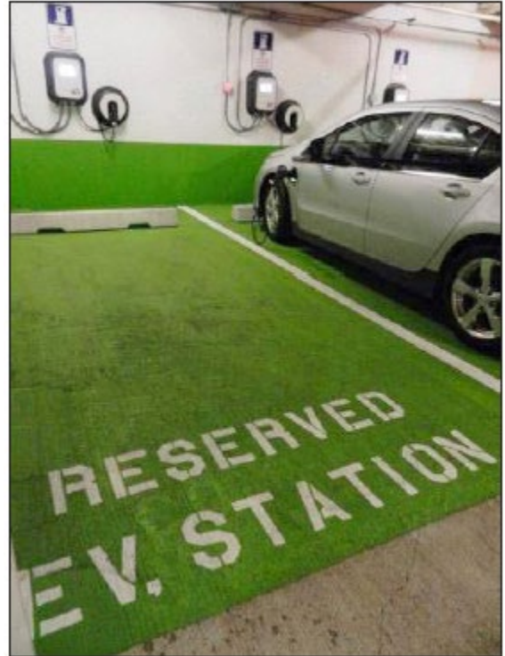
Figure 1 Example from City of Madison's notice on EV Ready / EV Installed requirements for Parking Facilities
