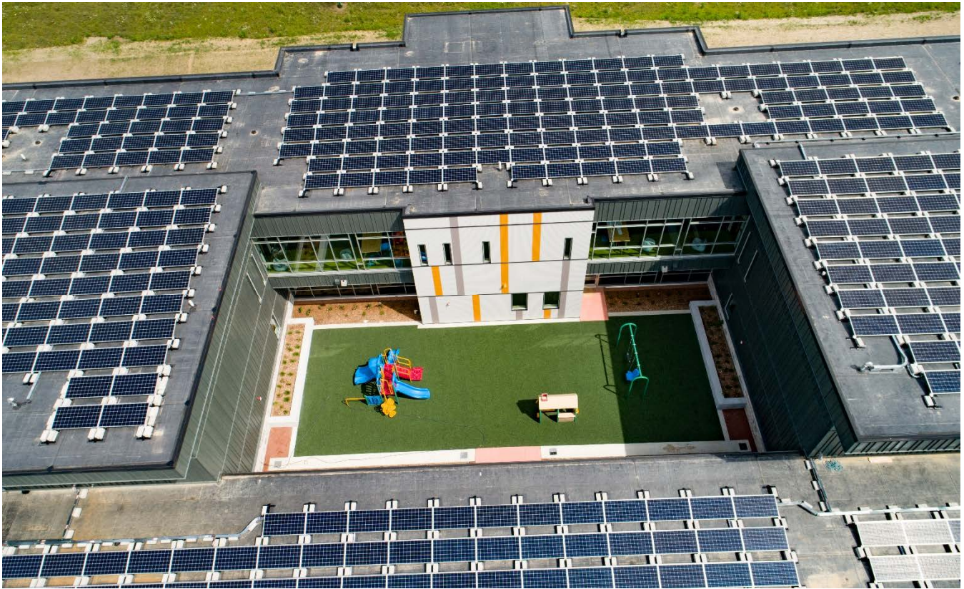
Figure 6- Closer image of solar PV panel and racking arrangement - similar design assumptions have been made for the new PSB project
