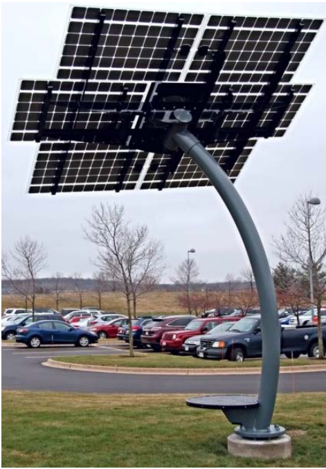
Figure 9- A more decorative example of ground mounted solar
