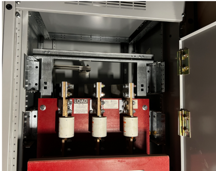
Main Switch Section
