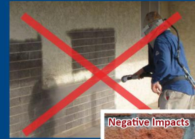
NOT PERMITTED Sandblasting can be very destructive to historic masonry, as shown above.
