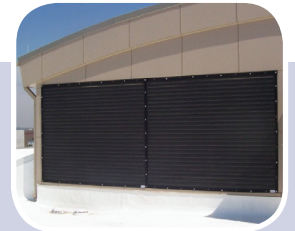
Louver & AHU Intake Filters
