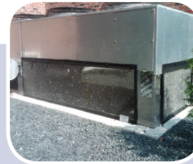
Dry Cooler Filters
