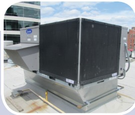
RTU Filters & Hail Guards
