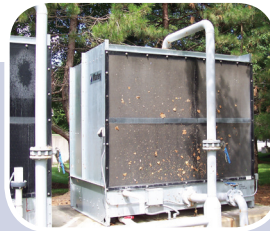
Cooling Tower Filters
