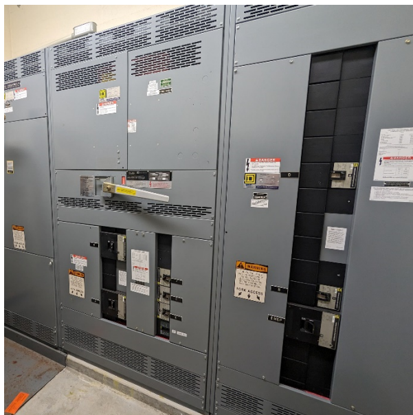
Figure 9- Existing main service panel is likely too small for the NZE electrical systems and generation
