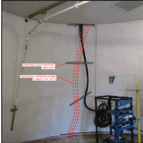
A COAX ROUTING (TANK BASE)
