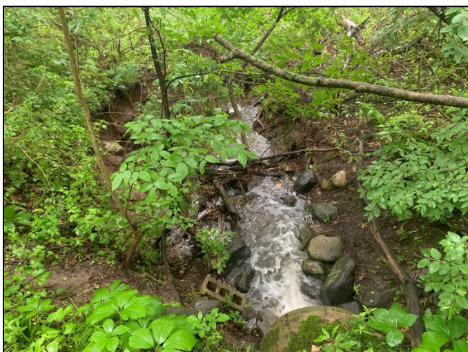
Photo 29. Severe gully erosion downstream of stormwater discharge pipe in Thrun Marsh Conservancy (large precipitation event on June 8, 2022).
