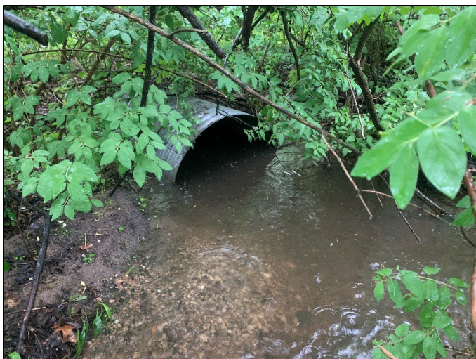
Photo 31. Culvert under the trail at terminus of severe gully erosional feature. View from the alluvial fan at the edge of Thrun Marsh (large precipitation event on June 8, 2022).
