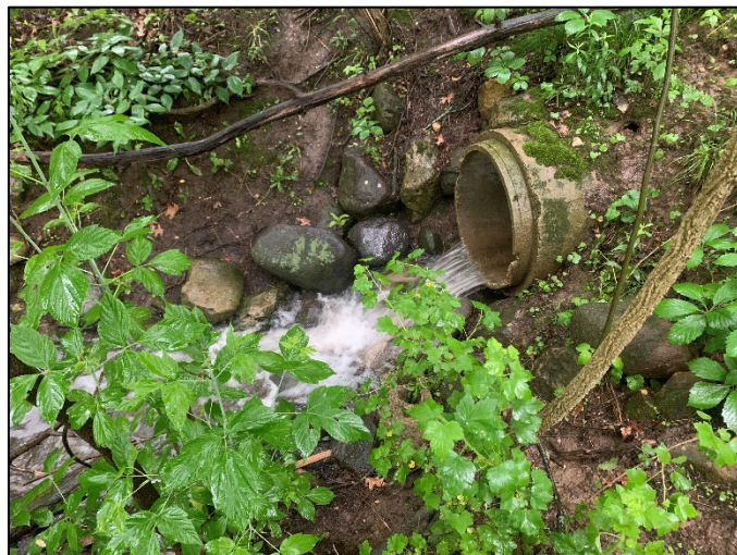
Photo 28. Stormwater discharge at pipe at upstream end of severe gully erosion in Thrun Marsh Conservancy (large precipitation event on June 8, 2022).
