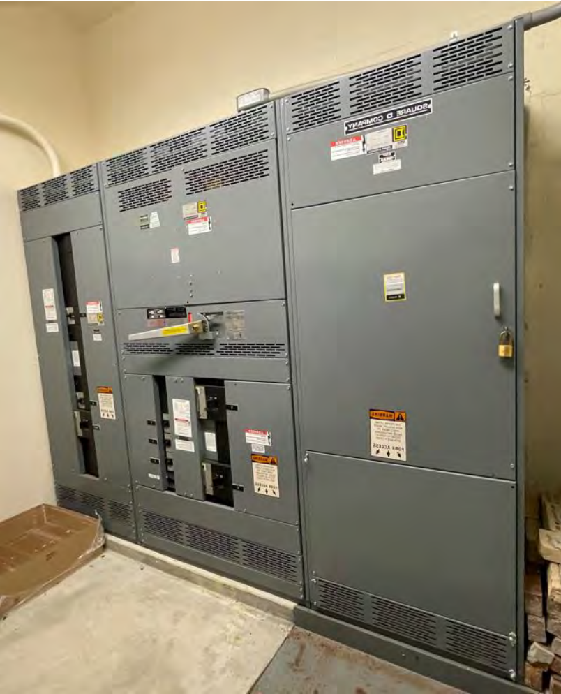
Figure 23: Existing Service Entrance Equipment
