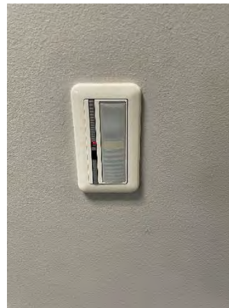
Figure 20: Existing Wall Occupancy Sensor
