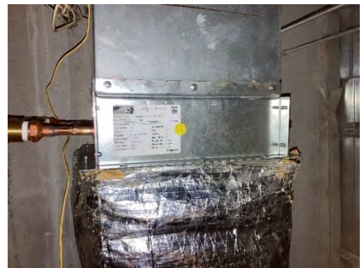
Figure 2: Hot Water Coil for VAV-4.02
