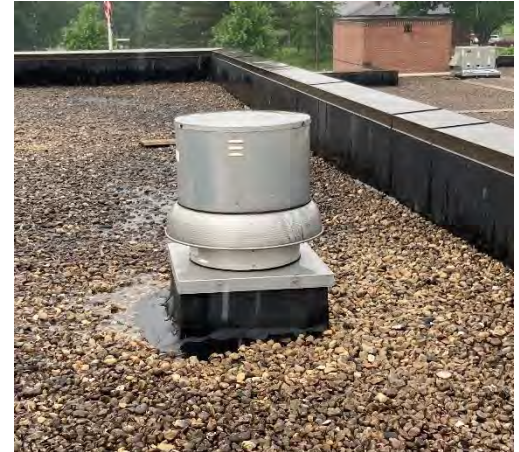
Figure 4: EF-5, visible corrosion. Carnes Downblast Exhaust Fan.
