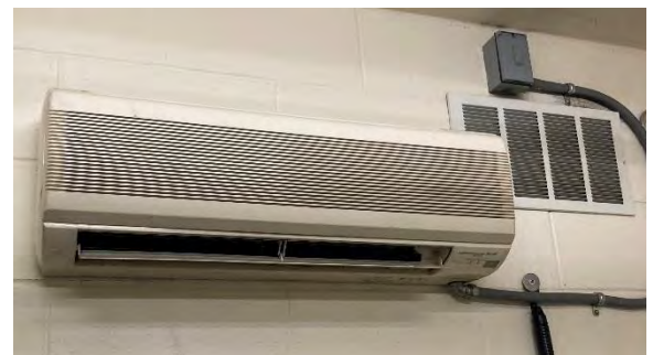
Figure 12: Mitsubishi Split System Heat Pump
