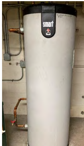
Figure 14: GWH-3, Operational Water Heater
