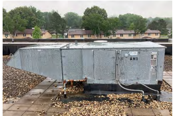
Figure 5: MAU-1, Fire Garage Make Up Air Unit.
