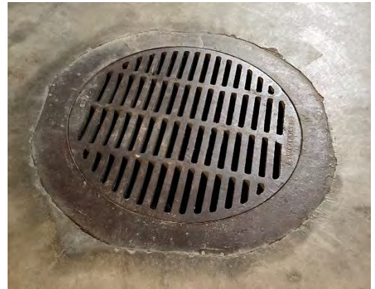
Figure 17: Garage Catch Basin
