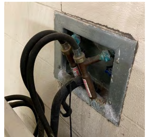
Figure 15: Visible Corrosion Example, Washer Box
