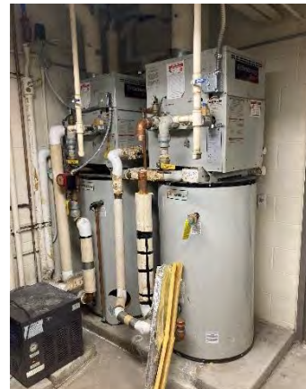
Figure 13: GWH-1,2 Decommissioned Water Heaters
