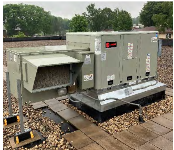
Figure 6: RTU-2, Trane Rooftop Air Handling Unit.
