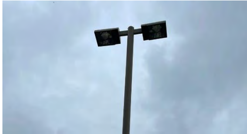
Figure 21: Existing Outdoor Light Pole
