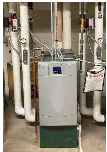
Figure 10: Peerless Boiler B-1
