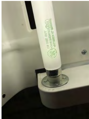
Figure 18: Existing Fluorescent Tube
