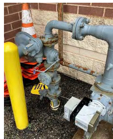
Figure 16: Rusting Gas Meter
