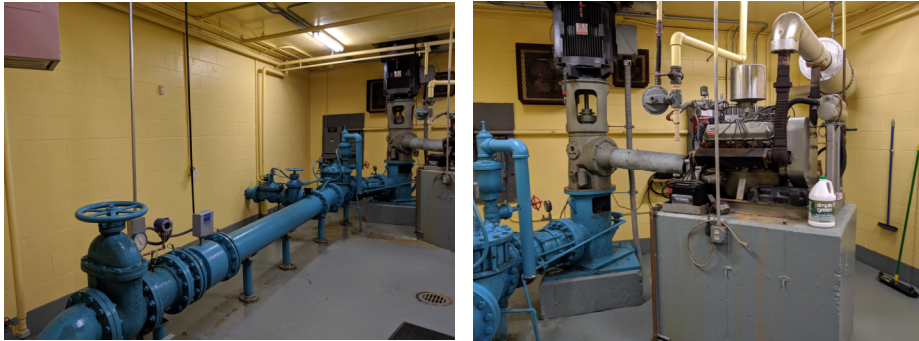
Well 4 Wellhouse Interior
