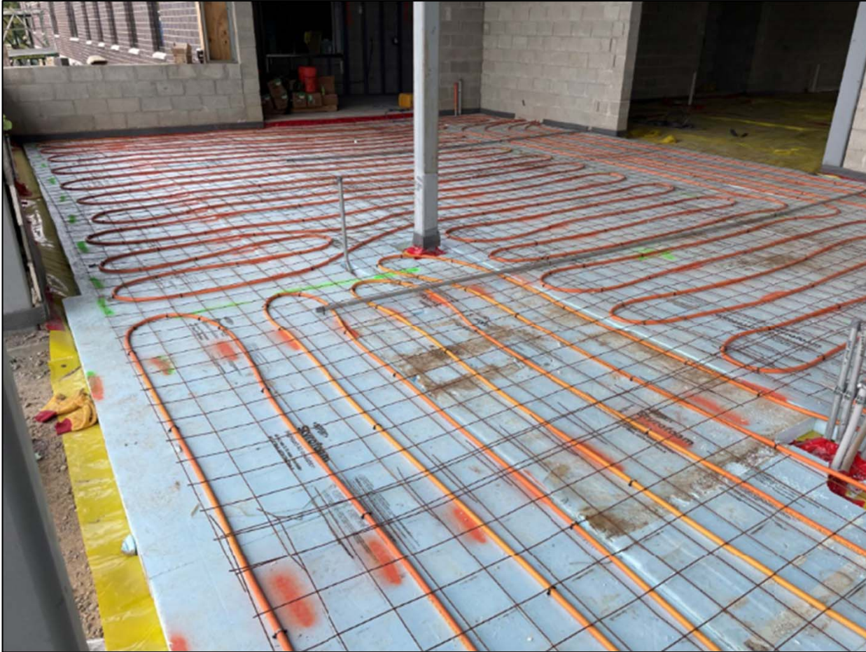
Radiant Tubing at Main Lobby
