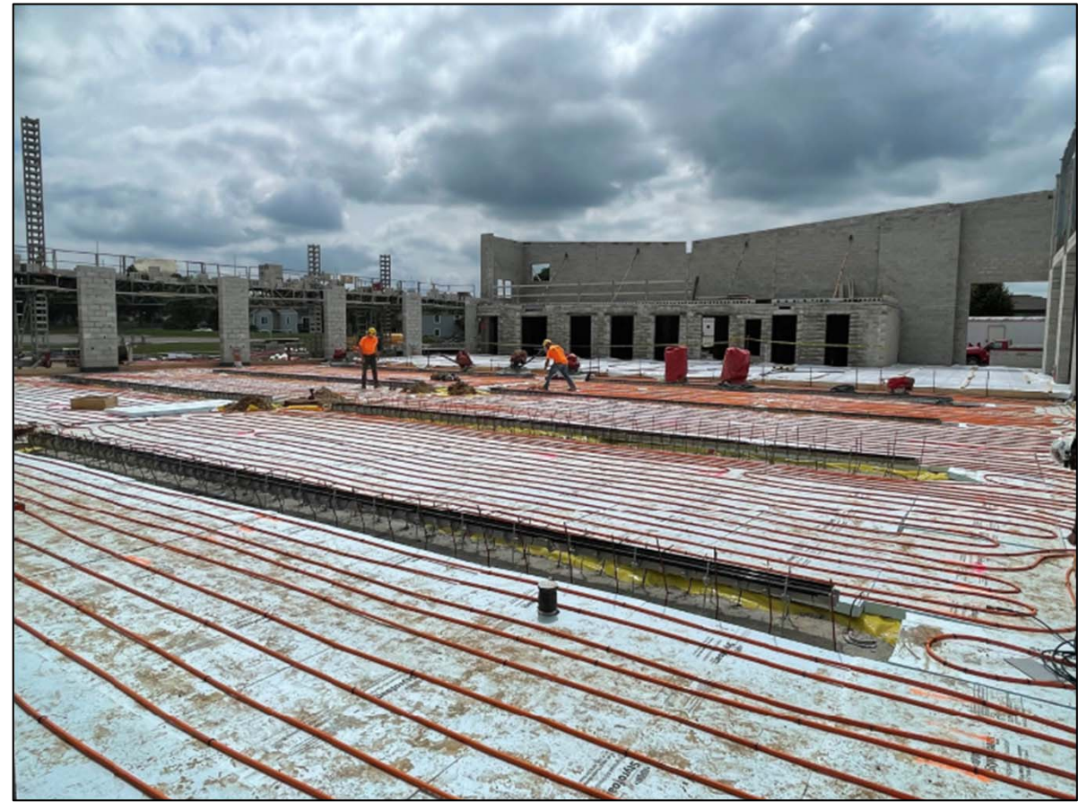
Radiant Floor Heating in the Apparatus Bay
