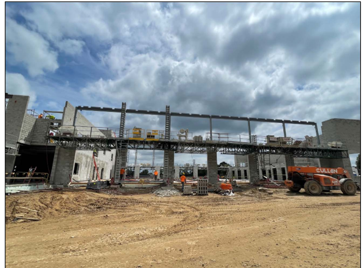
Masonry at Apparatus Bay Entrances
