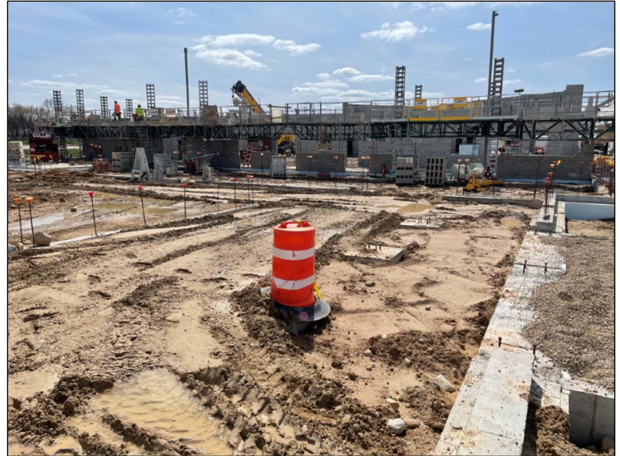
Lobby and Clerk area (foreground) Fire Unit (background)
