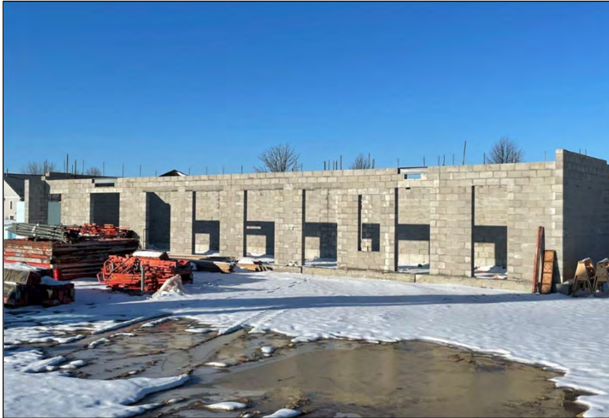
Masonry at Fire Unit Turn-Out Gear
