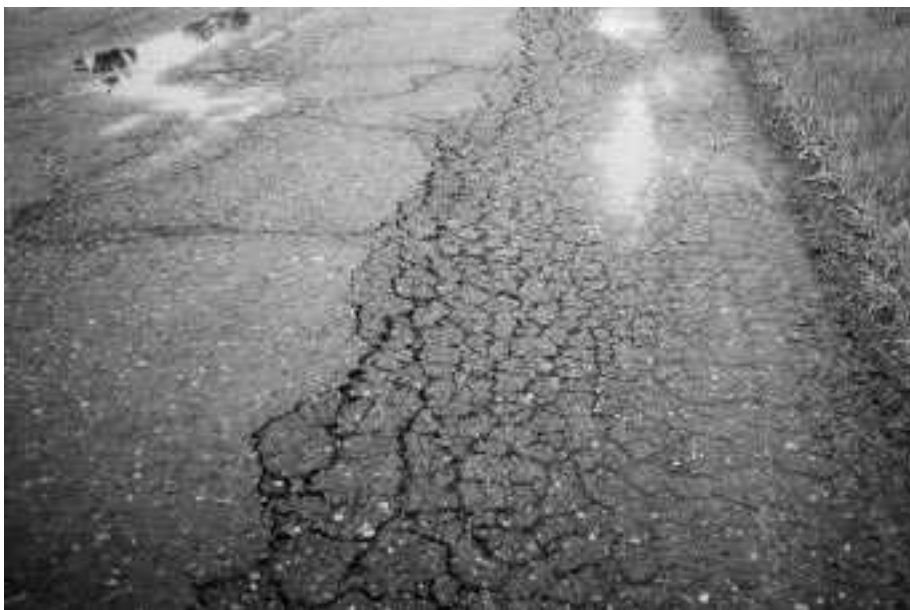
◀ Open raveled alligator cracking with settlement along lane edge most likely due to very soft subgrade.
