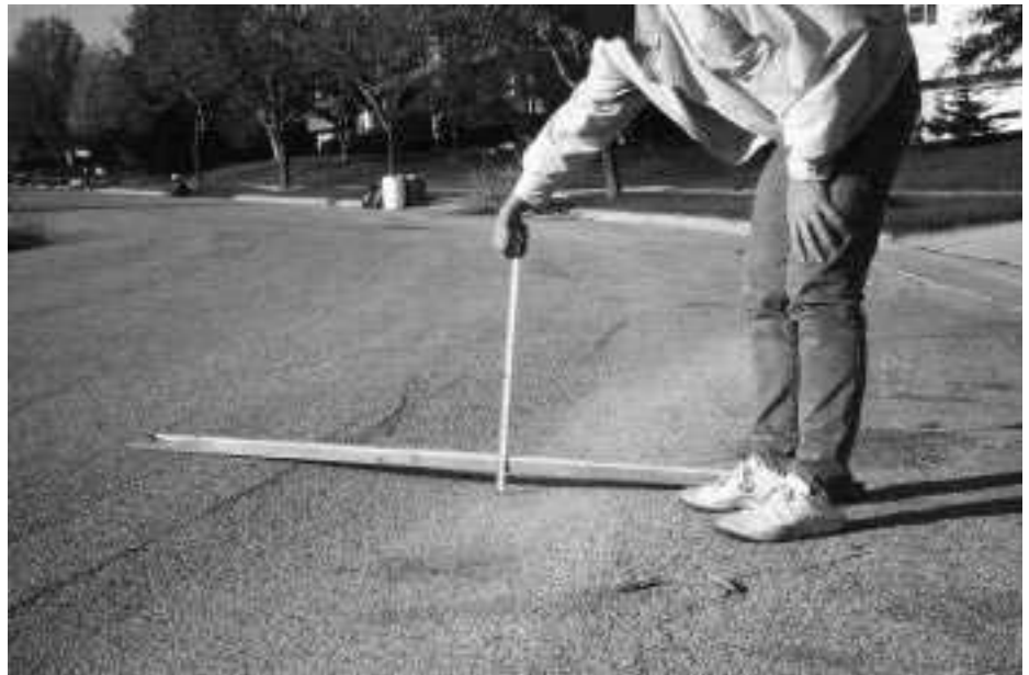
► Severe settling from utility trench.
