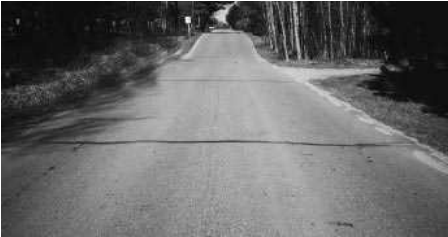
▼ Widely spaced, well-sealed cracks.
