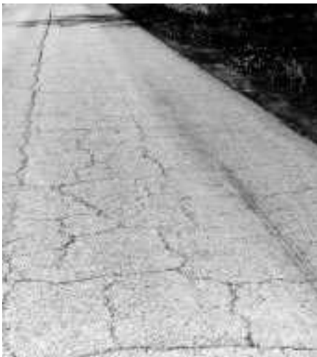
▲ Extensive block cracking in an irregular pattern.
