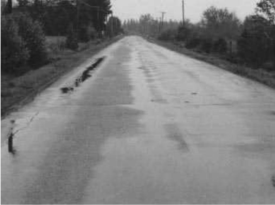
◀ Even slight rutting is evident after a rain.
