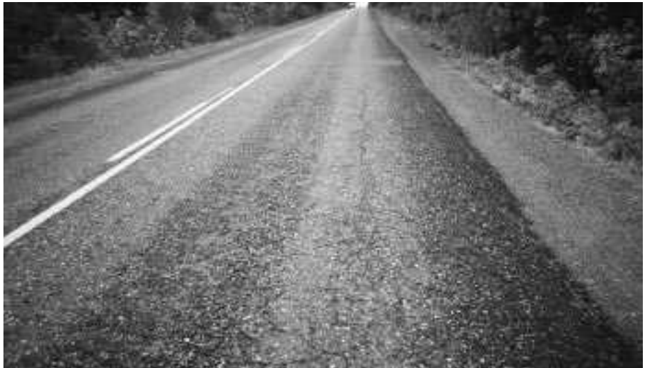
► Moderate to severe raveling in wheel paths.
