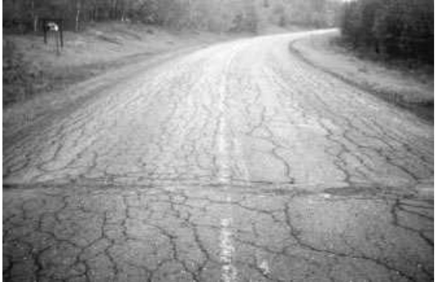
▶ Extensive alligator cracking. Pulverize and rebuild.
