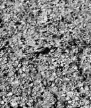
Severe raveling with ▼ extreme loss of aggregate.
