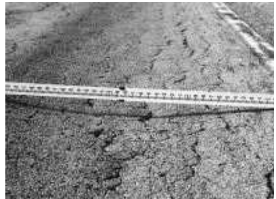
▲ Severe rutting. Strengthen base and reconstruct.
