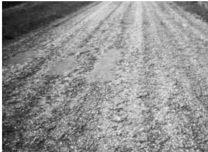
◀ Severe raveling and loss of surface material.
