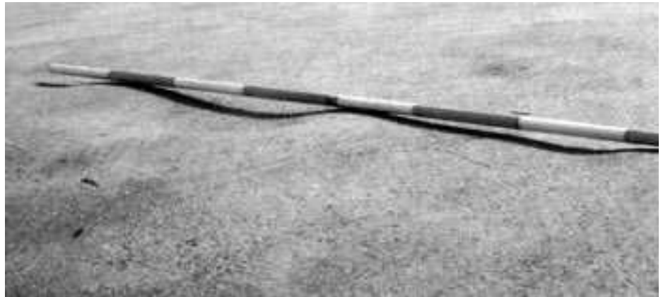
▼ Heavy traffic has shoved pavement into washboard ripples and bumps.
