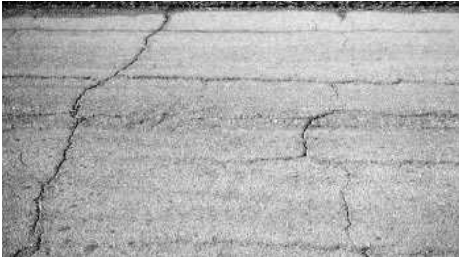
▼ Block cracking with open cracks.
