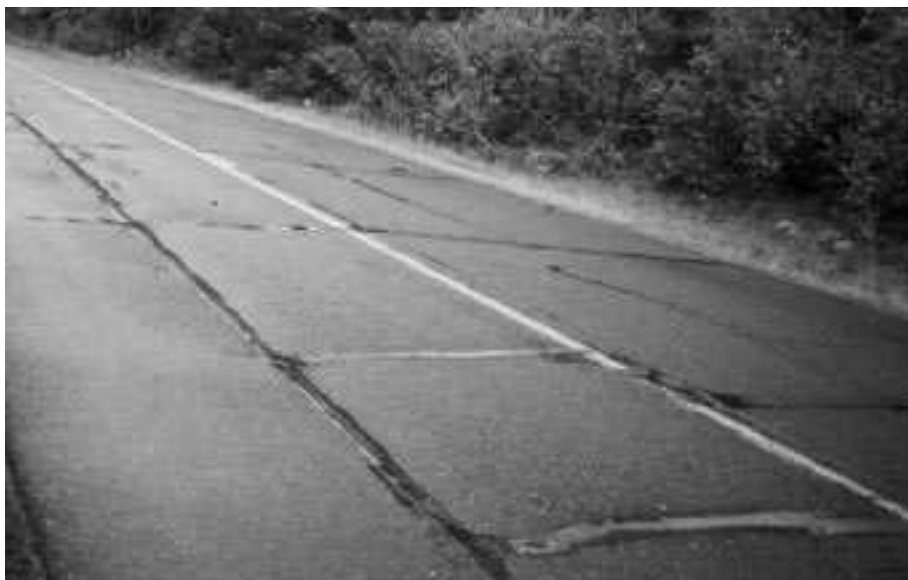
► Concrete joints reflected through bituminous overlay.
