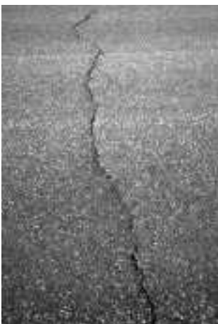
▲ Tight cracks less than 1/4" in width.
