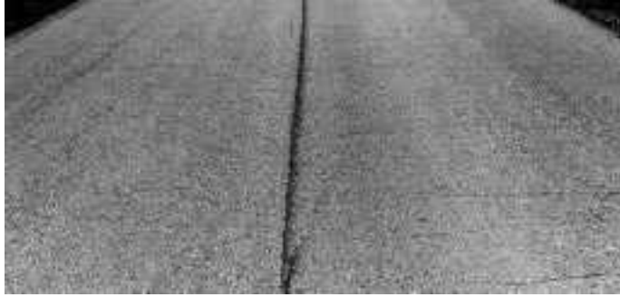
Centerline crack (still tight). ▶
