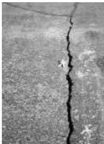
▲ Open crack – 1/2" or more in width.
