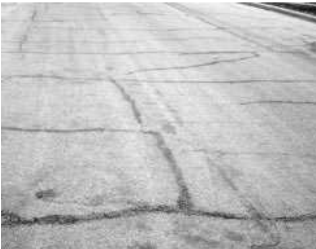
▼ Large blocks, early signs of raveling and block cracking.
