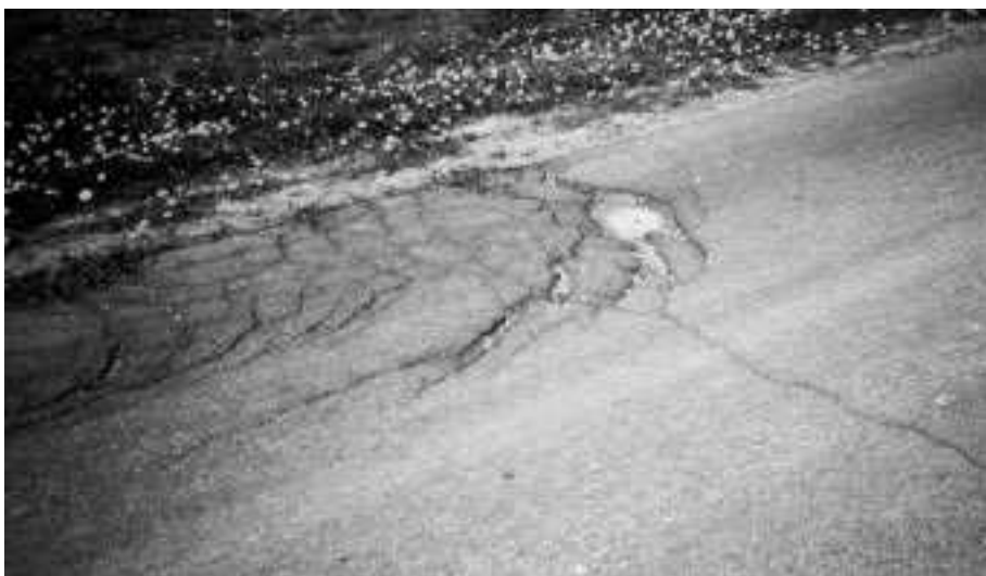
► Crescent-shaped cracks characteristic of slippage.
