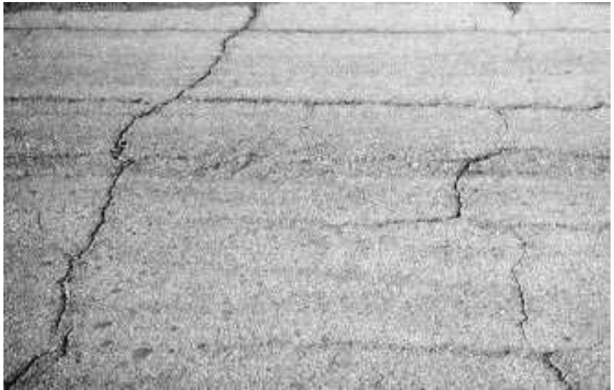
▶ Intermediate-size block cracking, 1'-5' across with open cracks.
