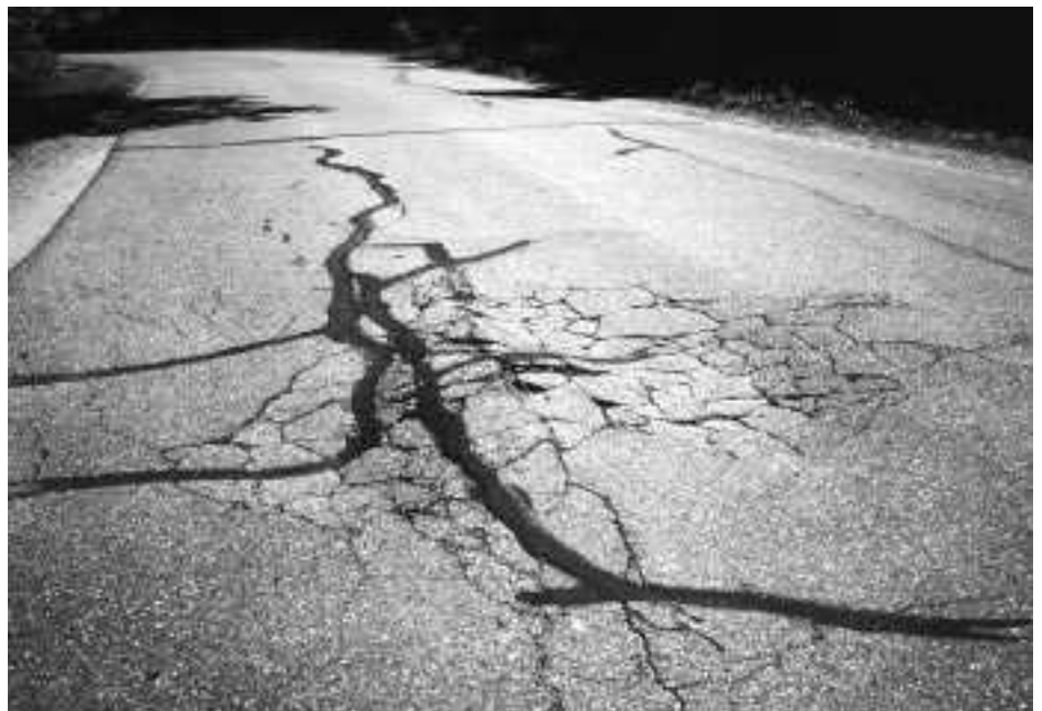
► Frost heave damage from spring break-up.
