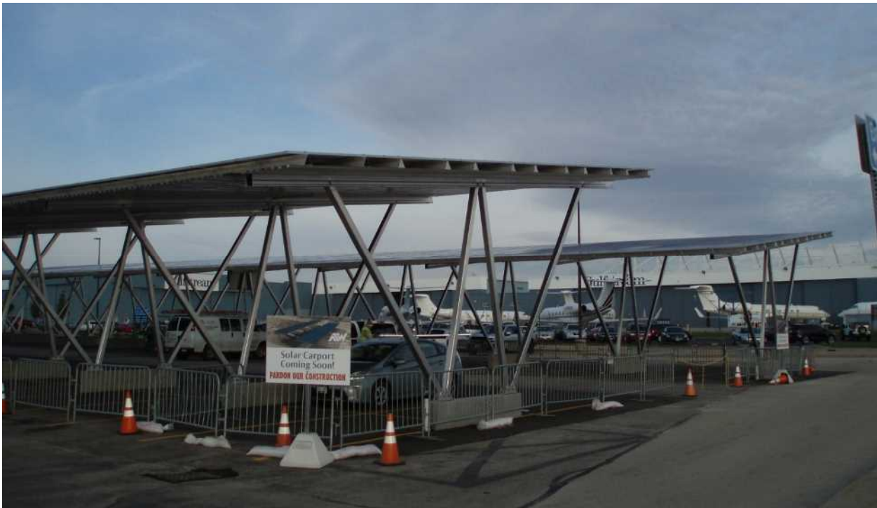
Figure 13- Example solar carport in Wisconsin
