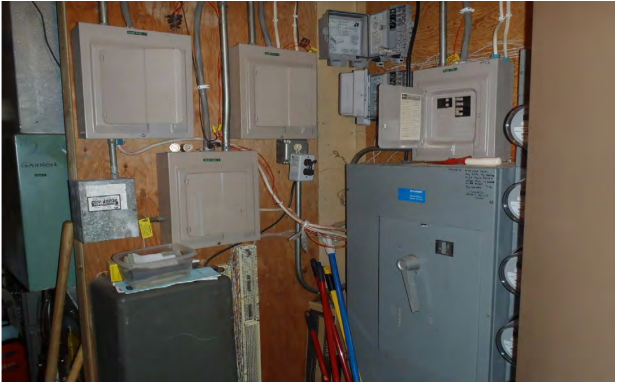
Photo 5 – Mechanical Room electrical panels.
